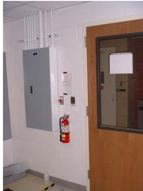
Fire extinguisher and LAMP emergency push button to the left of lab entrance door
