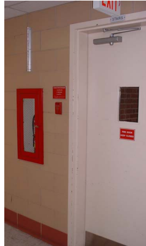
Additional fire extinguisher and fire alarm pull station in front of LAMP exit door
