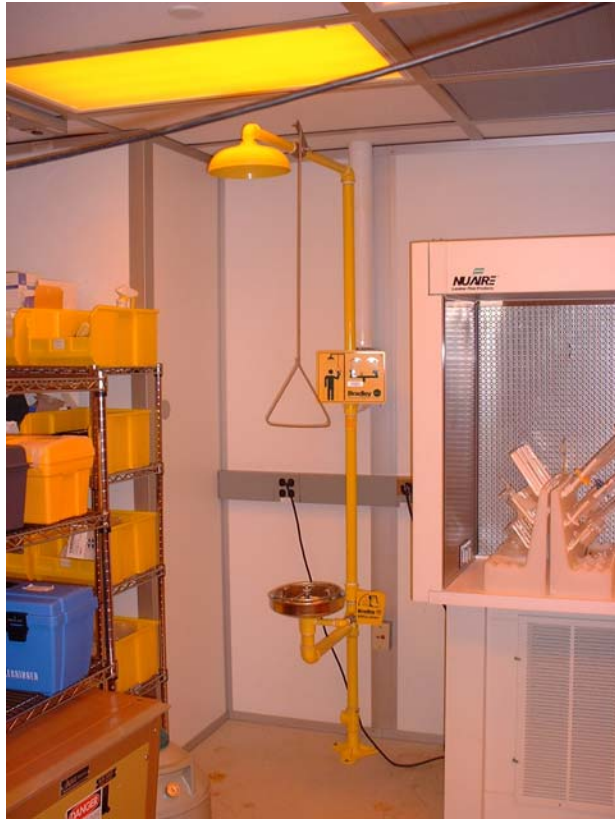
Eye wash station and emergency shower (40 gal/min) in left back end corner of cleanroom
